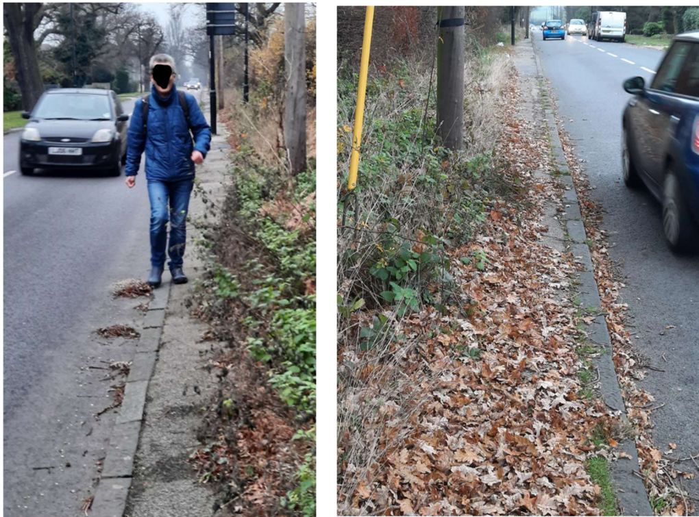
Figure 59: narrow and obstructed footpath along Waggon Road (no pavement on other side of road) (Source: HWNPF)
